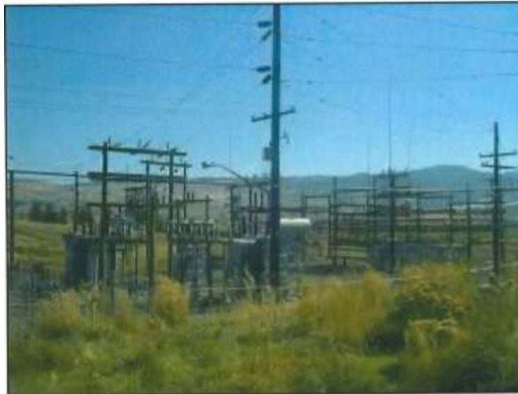
Figure 3 – Power substation near Merritt, BC
