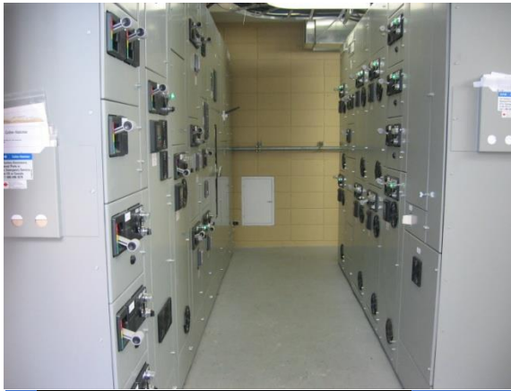
Motor Control Centre
