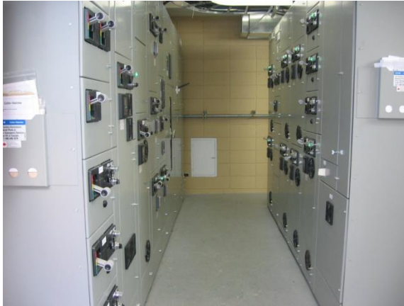
Motor Control Centre
